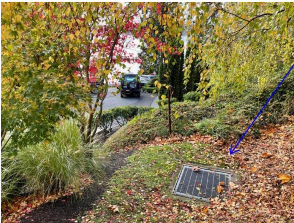
PS 20 – Generator Enclosure
